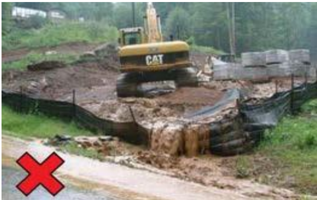
Figure 10: Silt fence failure
